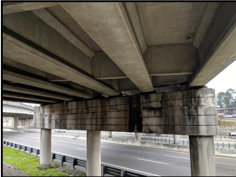
5 Tar material located on east side bents test negative for asbestos via PLM and TEM analysis.
