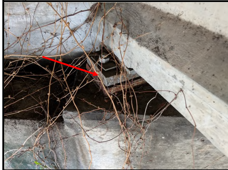
4 The vibration dampeners tested negative for asbestos via PLM and TEM analysis. The gray bent plate tested positive for lead-based paint (23.90 mg/cm 2 ).
