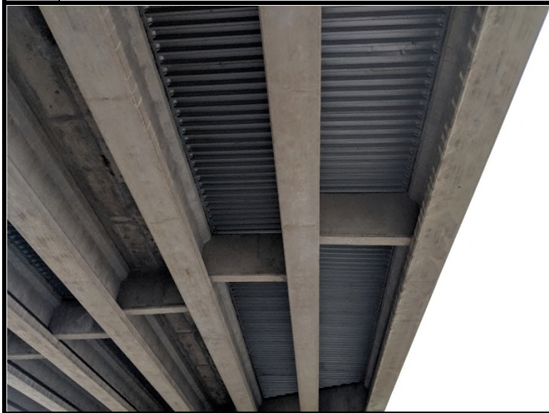
3 View of the underside of the bridge. Shows concrete beams and metal decking on the west side of the bridge.
